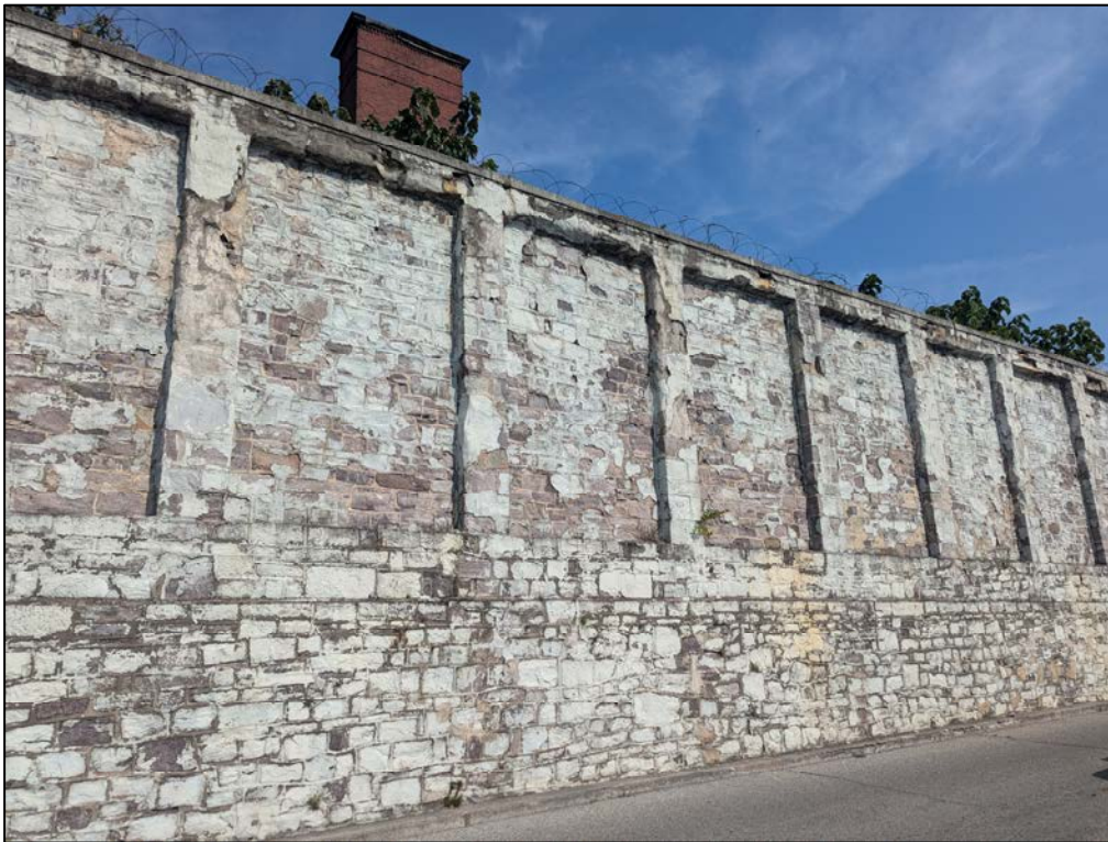
Figure 8. Maris Street perimeter wall showing spalling, west elevation
