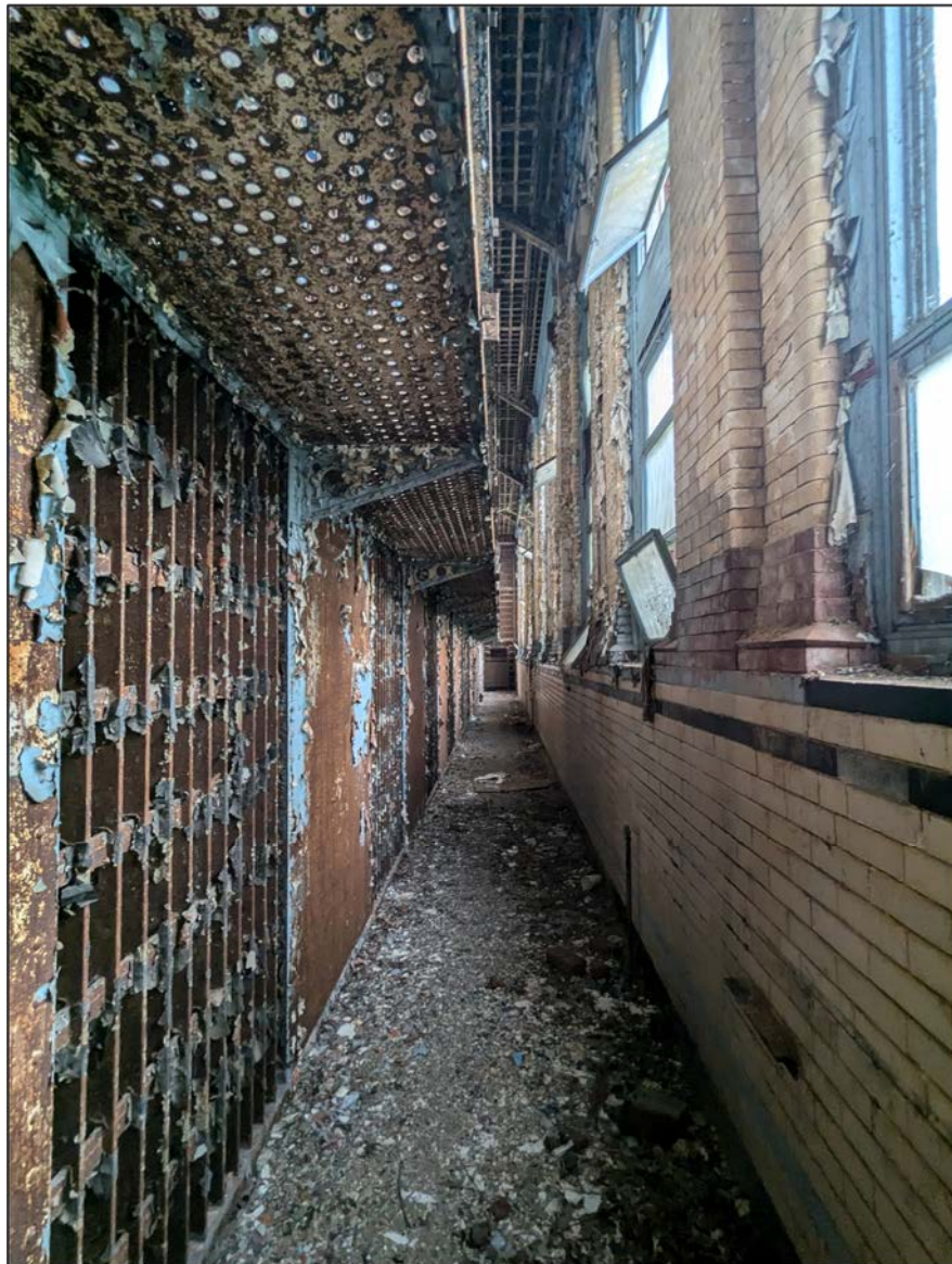
Figure 18. View of corridor between steel cell structure and brick building exterior wall
